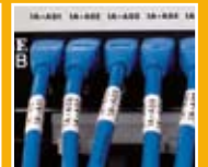
Perfectly Spaced Patch Panels
