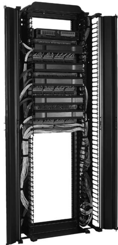
Vertical and horizontal cable managers work together to make an orderly installation
