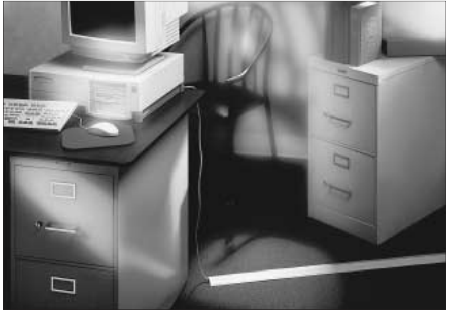
The Corduct Overfloor Cable Protection System in use in a typical office installation.
